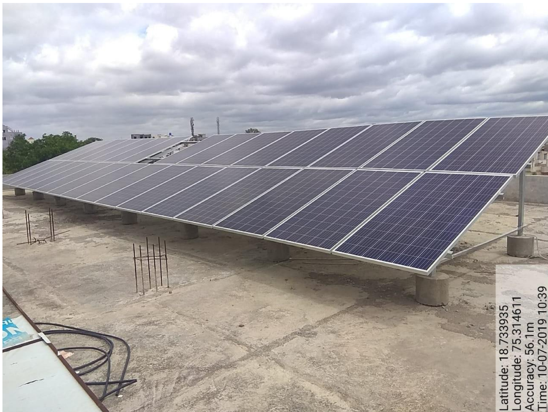
Photo-4: 10 kW solar roof top on institute building roof.
