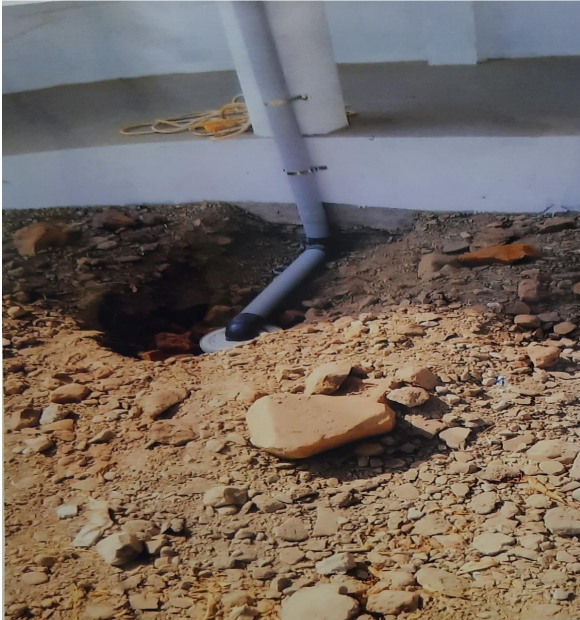
Photo-5: View of pipe for rain water collection from building
